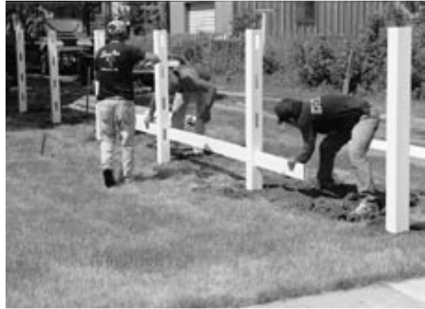
Threading the first rails, starting at the bottom. If spacing permits, rails are staggered at the joints.
